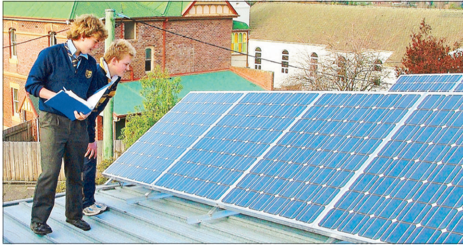
ALTERNATIVE POWER: St James Catholic College has installed Solar Panels to help reduce bills and minimise their global footprint.
